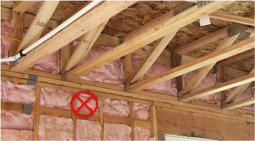
This photo shows rim joists that have been insulated. Unfortunately, the work is too sloppy to meet QII. There is too much compression and there are too many voids.
